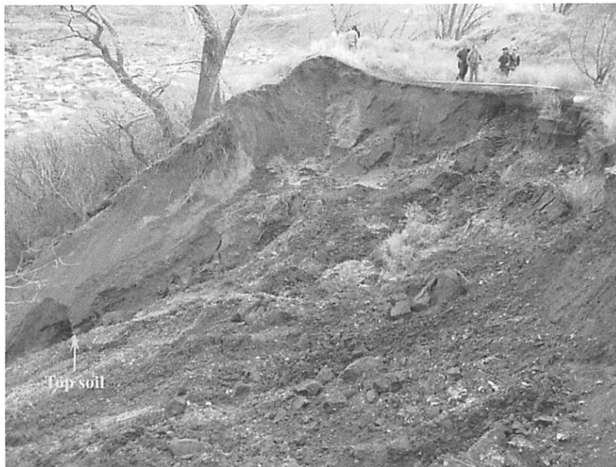
Figure 6. View to the southeast showing landslide main scarp and fill placed on the upper slope. Near the left edge of the photo, black top soil at the base of the scarp (arrow) underlying the brown fill is evident and indicates the original slope surface.
