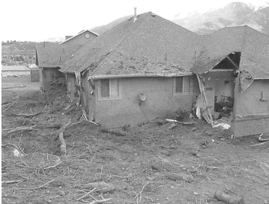
Figure 4. Damage to the house and garage at 1650 East 7687 South.
