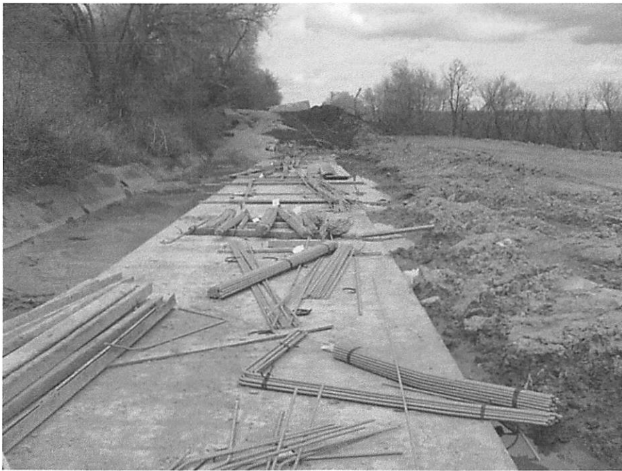
Figure 9. View looking northwest of Davis-Weber Canal showing landslide material deposited on the box culvert and canal access road. Following the landslide water and sediment flowed into the canal left of the box culvert.
