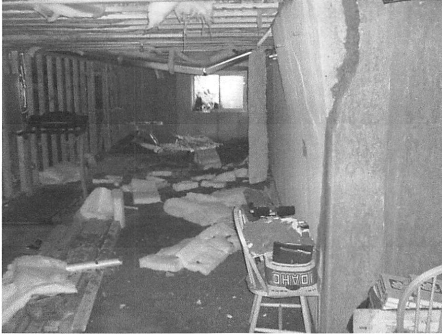
Figure 8. Basement at 1650 East 7687 South showing upper foundation wall (right side of photo) broken by landslide impact.
