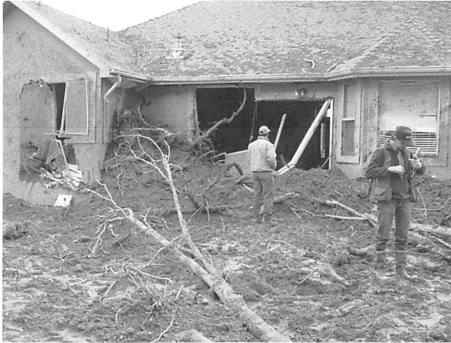
Figure 3. Landslide damage to the house at 1650 East 7687 South.
