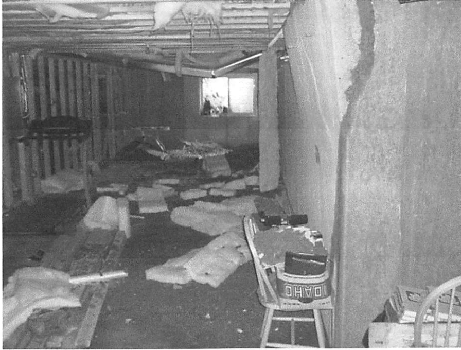
Figure 8. Basement at 1650 East 7687 South showing upper foundation wall (right side of photo) broken by landslide impact.
