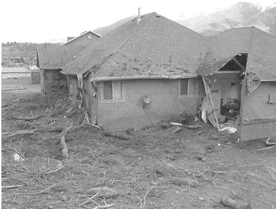
Figure 4. Damage to the house and garage at 1650 East 7687 South.
