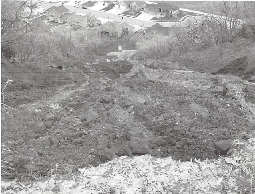
Figure 7. View looking down the landslide flow path at the damaged house at 1650 East 7687 South. The culvert in the lower slide path above the house was originally in the gravel pit. Subsequent water flow eroded the right side of the landslide.
