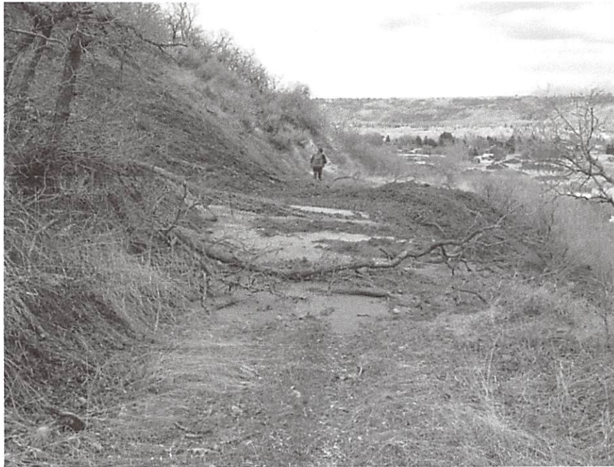
Figure 10. Landslide material deposited on a dirt road midslope above the Davis-Weber Canal.
